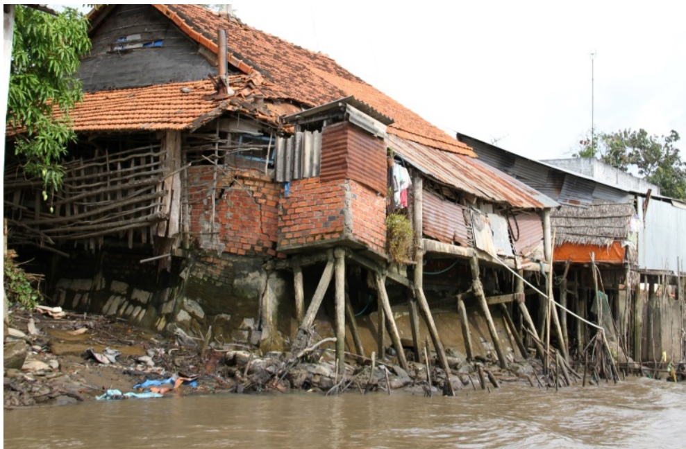
Figure 6: House in Ca Ma, Mekong Delta undermined by erosion. Source: (Natural Heritage Institute 2015).
